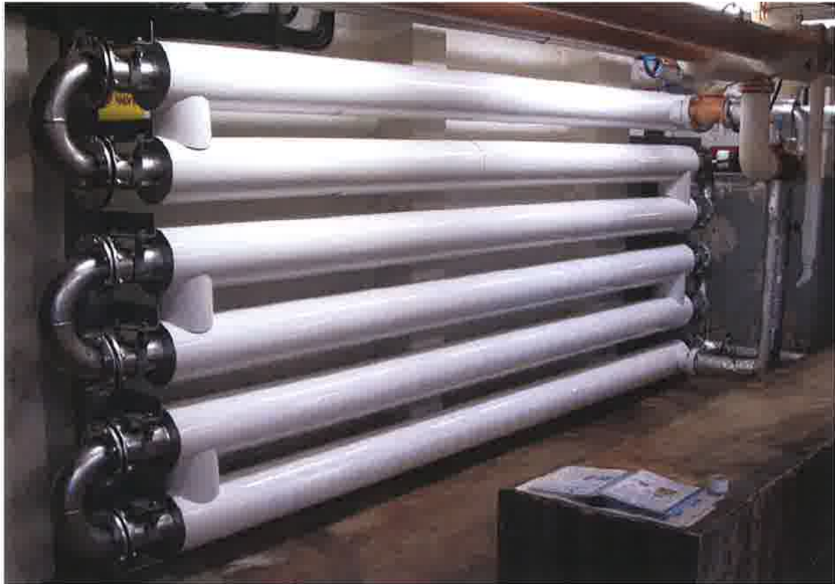
Figure 6 – Treated Effluent Heat Recovery System
