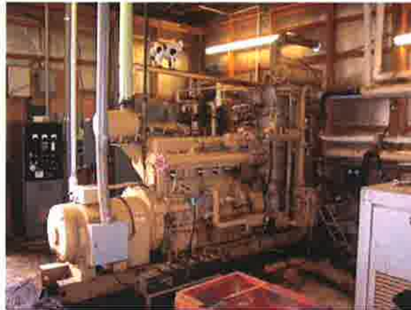
Figure 4 – Bio-Energy Cogeneration System
